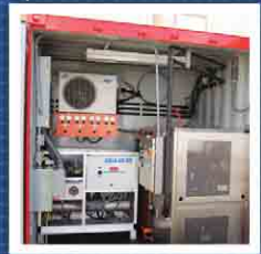
Equipment side of module
